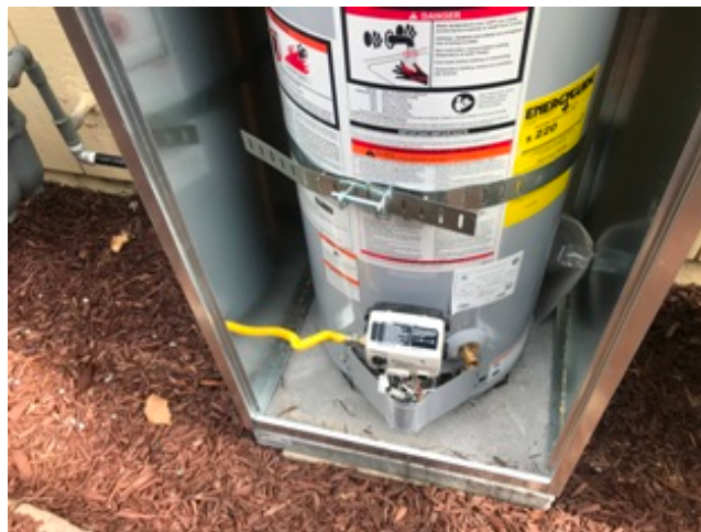
Unsafe Installation of Water Heater Gas Line
